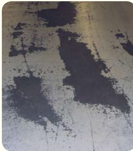
Eliminate Coating Failures
