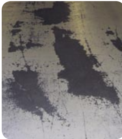
Eliminate Coating Failures
